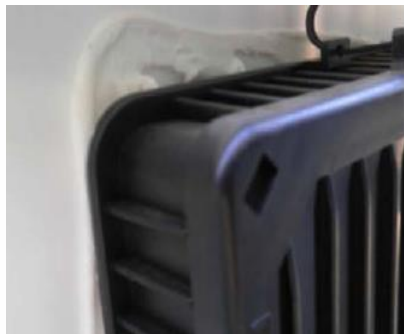
Junction box failure
