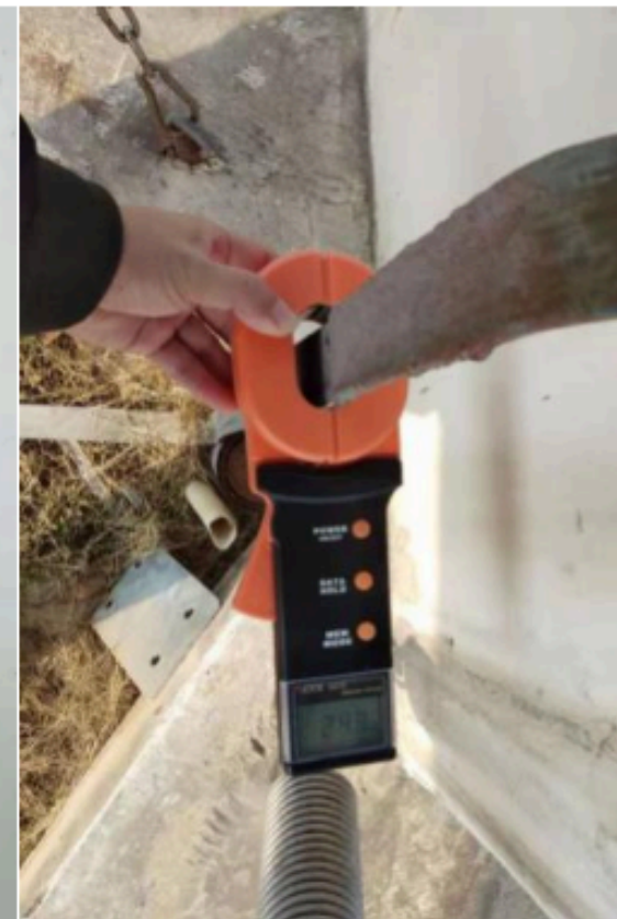
Poor system grounding
