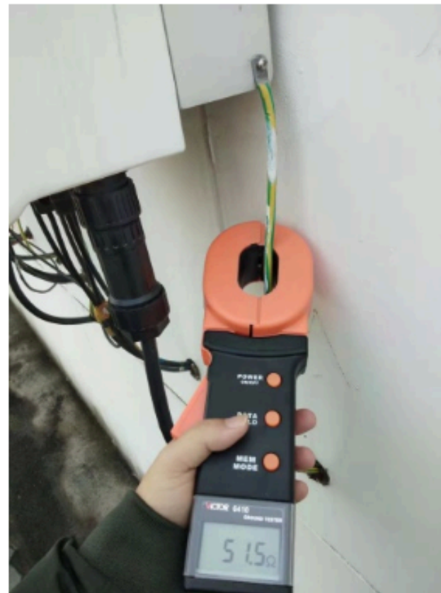
Poor inverter grounding
