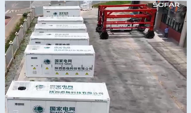
25 MW/50 MWh, Xian, China by China State Grid
