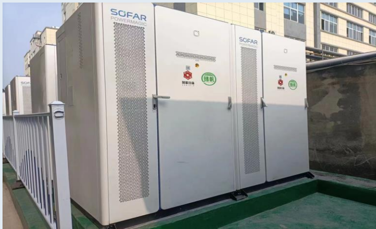
1.25MW/2.15MWh, Zhejiang, China
