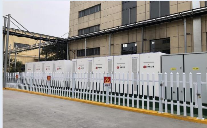
1MW/1.72MWh, Jiangsu, China
