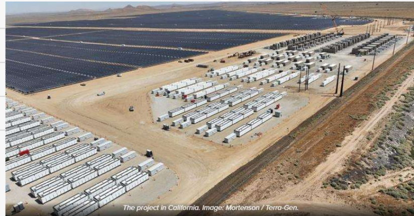
PV Edwards Sanborn: 875MW DC BESS: LG Chem, Samsung, BYD
